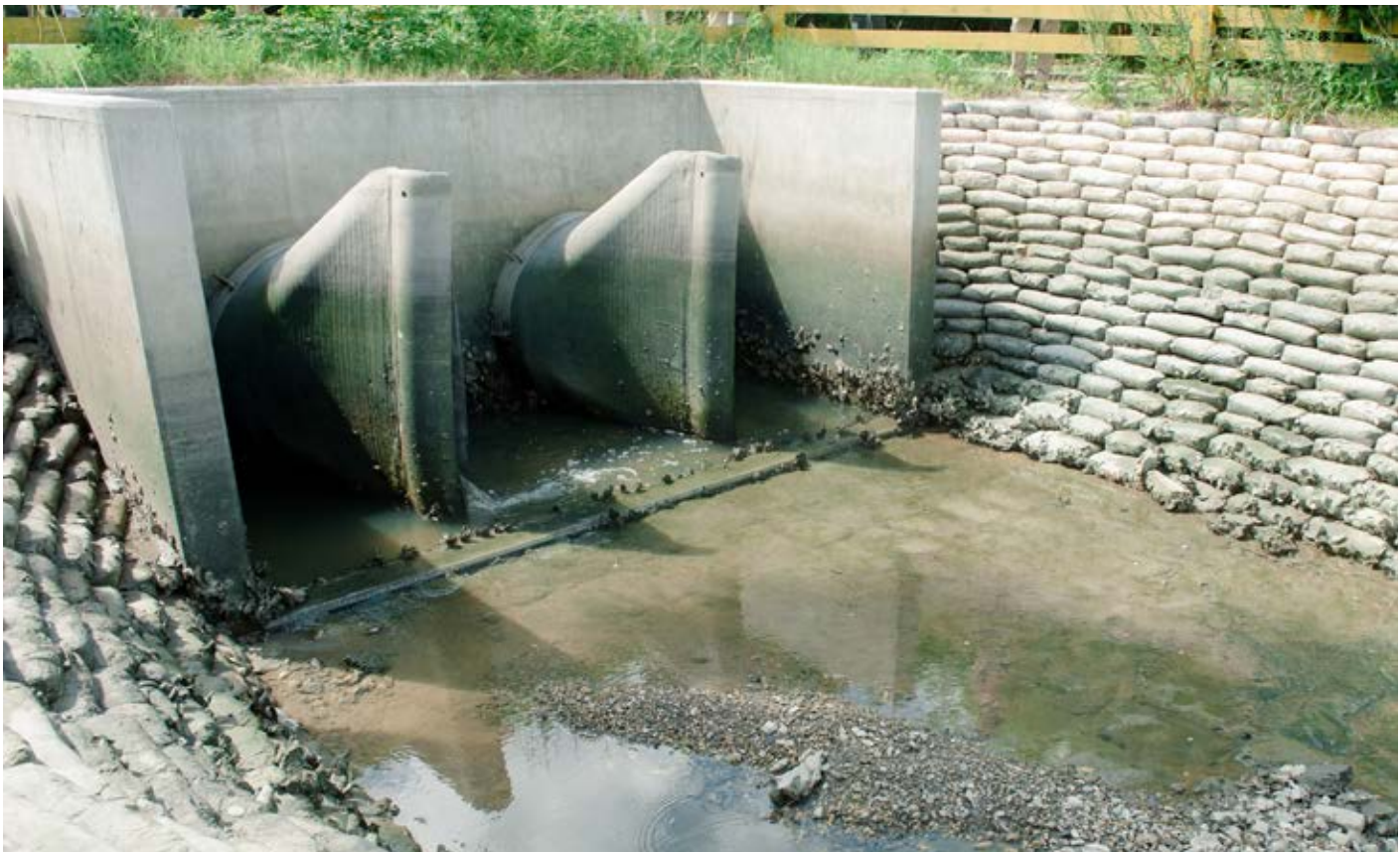
FIGURE 4.9: STORMWATER TIDAL BACKFLOW PREVENTERS, NEAR INTERSECTION OF 14 TH ST. AND VENETIAN DR.
